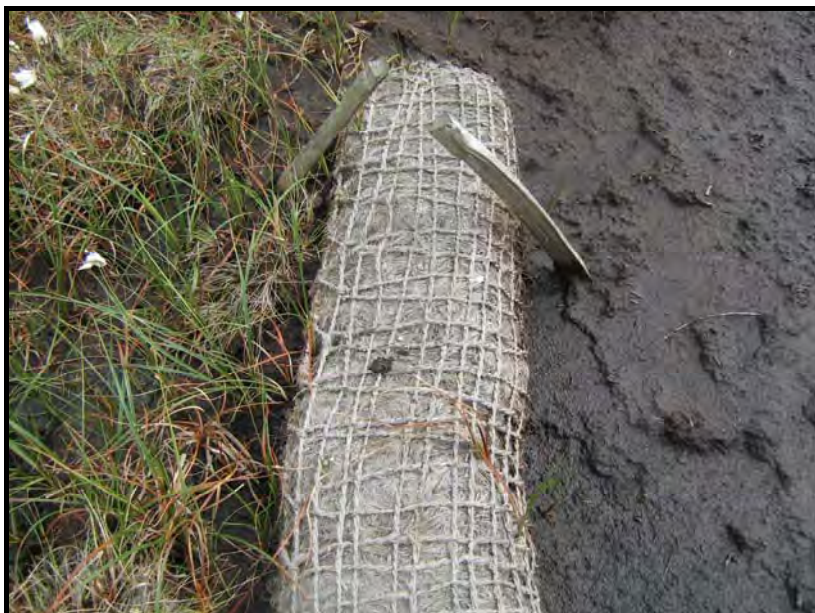
Photograph 17 Coir Roll on Ashway Gap Showing Peat Accumulating and Vegetation Colonising Behind the Coir Roll (Note the uneven surface of the exposed bare peat indicating the surface 'downstream' of the coir roll is still highly mobile and vegetation establishment is likely to be compromised)
