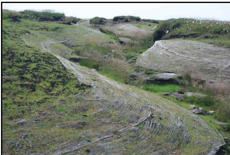
Photograph 16 Slope Stabilisation Using Geojute Matting (note the re-vegetation following addition of lime, grass and heather seed, fertiliser and heather brash)
